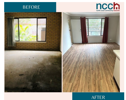
Before and After photos of the refurbishments done at the Laurel Lodge complex. Each unit had a new kitchen installed, new interior & exterior paint, new flooring and the balconies were repaired and painted.
